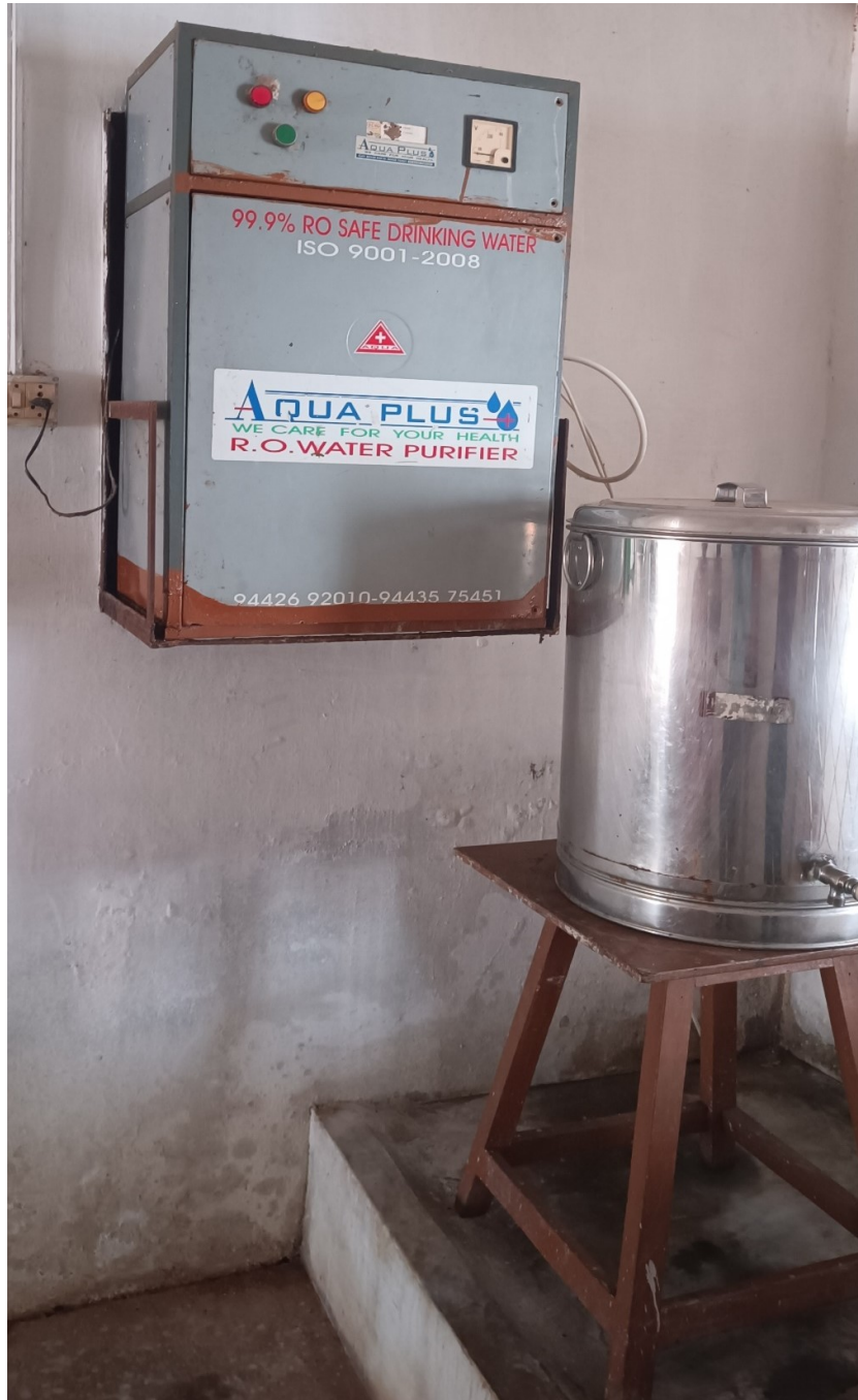
Fig.16. RO water plant at College & Hostel
