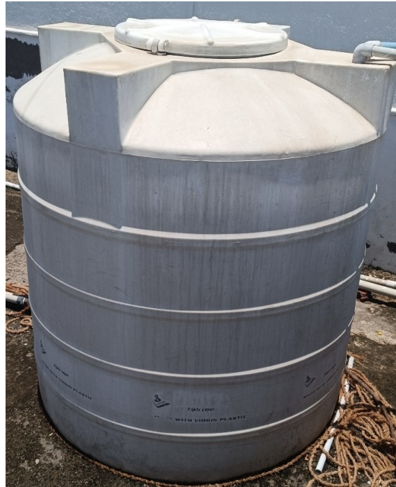
Fig. 13. Overhead sintex tank for RO plant
