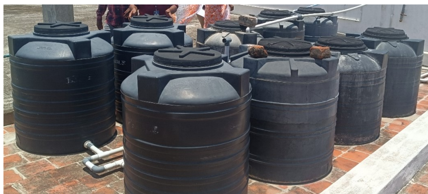
Fig.14. Overhead sintex tank for hand wash, toilet, other applications.
