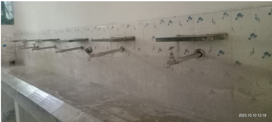
Fig.18. Fresh water distribution to Hostel.
