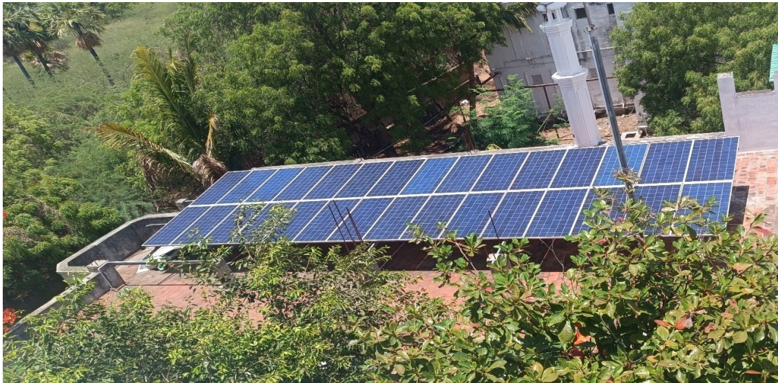
Fig.35. Installed 10kW solar PV plant at college rooftop.
