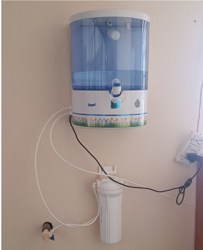
Fig.15. RO water plant at Library
